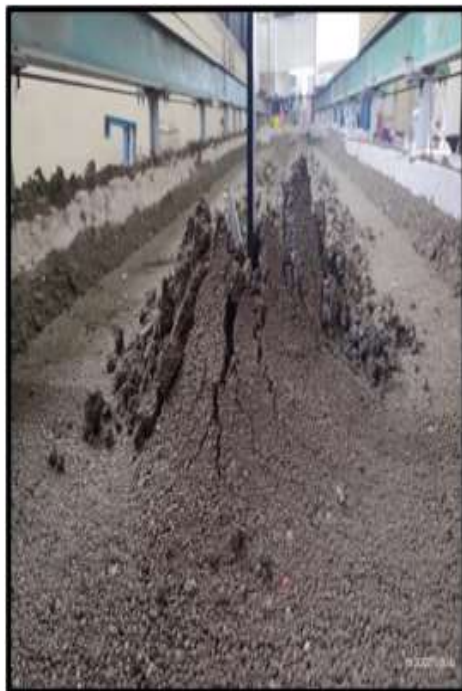
Plate 3a: Soil failure pattern
